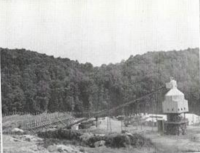
From huge storage bins gravel is sent up conveyor belt to concrete mixing tower.
