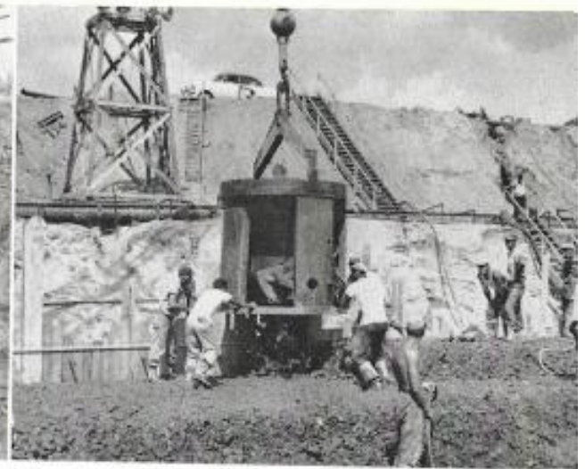
Bucket is opened and concrete pours out. Bucket is then swung back to truck for next trip.
